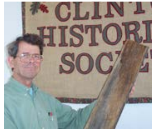
Dick Coller holds a rotted exterior sill board.
