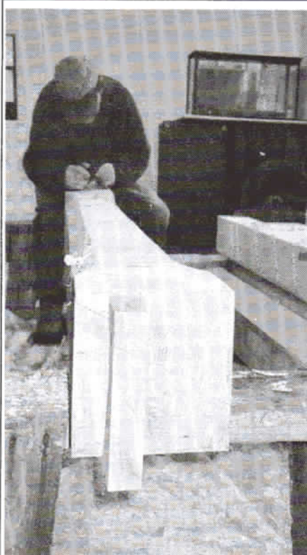
This is one of the timber framers working on the posts that are being reinstalled on the second floor of the Creek Meeting House.
